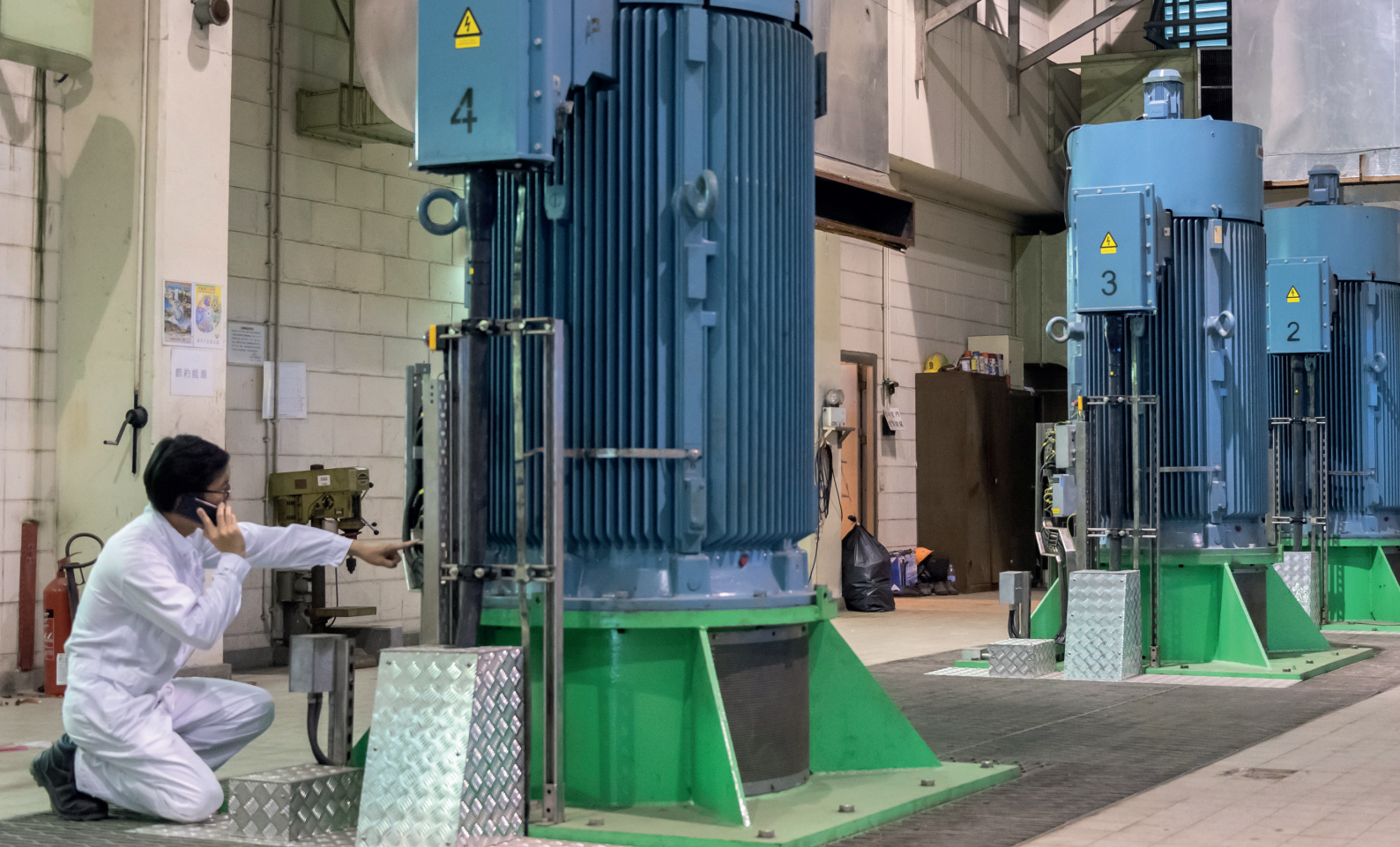
Sha Tin Sewage Treatment Project in Hong Kong, China. Photo: Asian Development Bank
